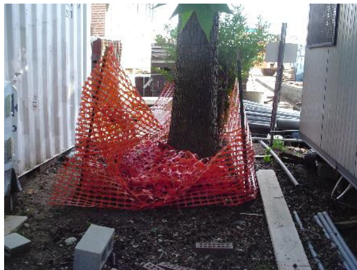
Figure 7: Inappropriate installation/maintenance of TPZ during construction
