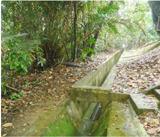
Perimeter Cut-off Drain along the staff quarters within Singapore Zoo
