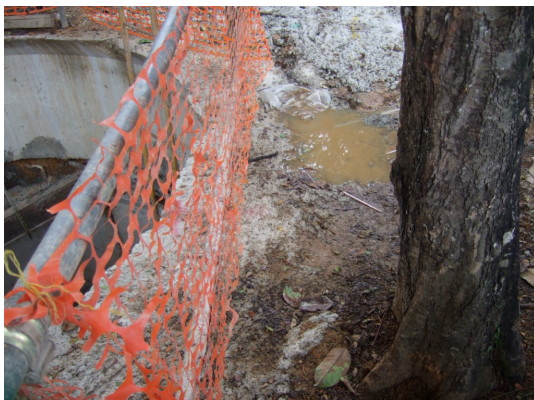
Figure 5: Construction cement deposited at tree base
